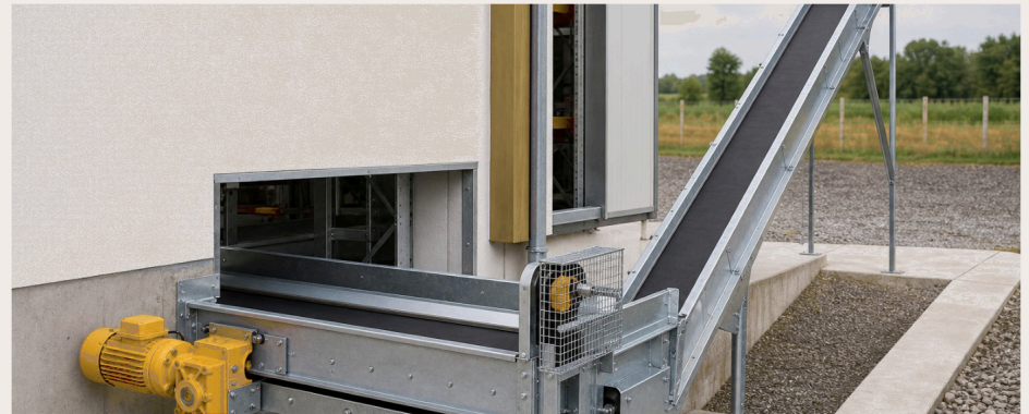
EXTERNAL DISCHARGE CONVEYOR
